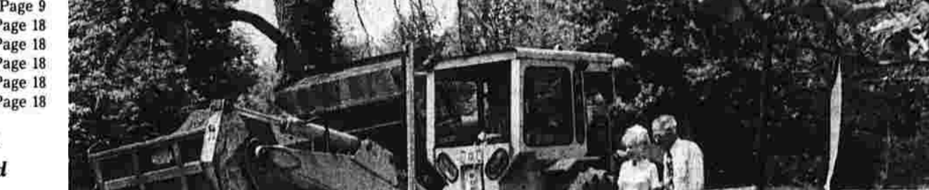
Men of the town highway department dig out the holes for the footings of the one-room schoolhouse to be located here on the grounds of the Cheney Homestead of Hartford Rd.
